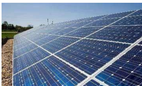
Figure 2 – Typical Photovoltaic Array
